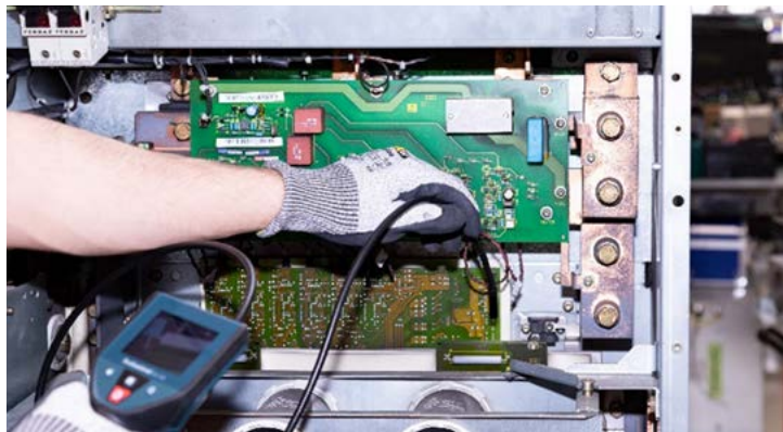
Fig. 2: Diagnosis and repair of power electronics control systems
